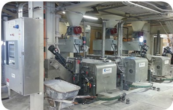
Davis WTP, Austin TX
