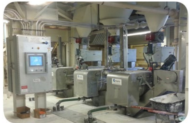
Davis WTP, Austin TX
